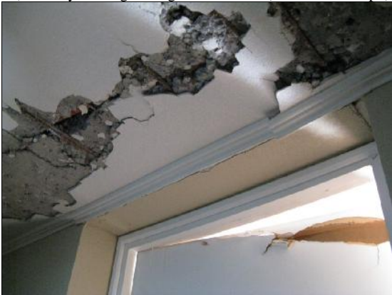
c) Damage due to wall/slab interaction
