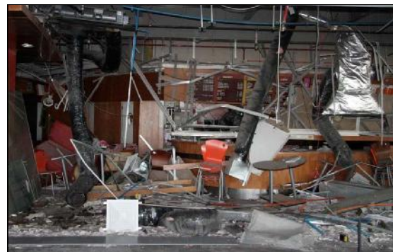
Figure 7. Example of generalized damage to non-structural components and systems (Miranda et al., 2012).
