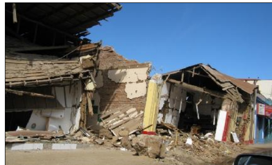
Figure 3. Typical damage non engineered structure.
