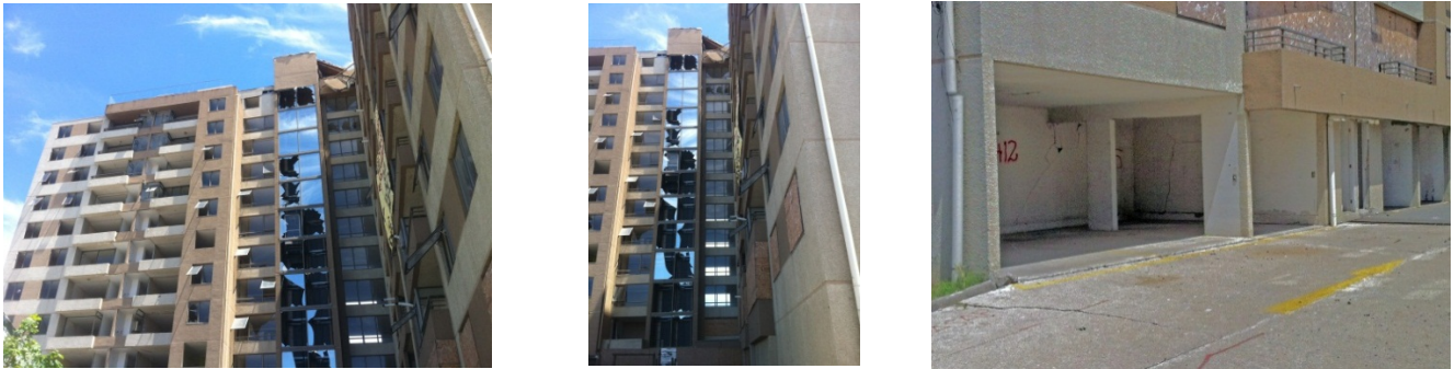
Fig. 4 - Damage observed in 12-storey reinforced concrete building
