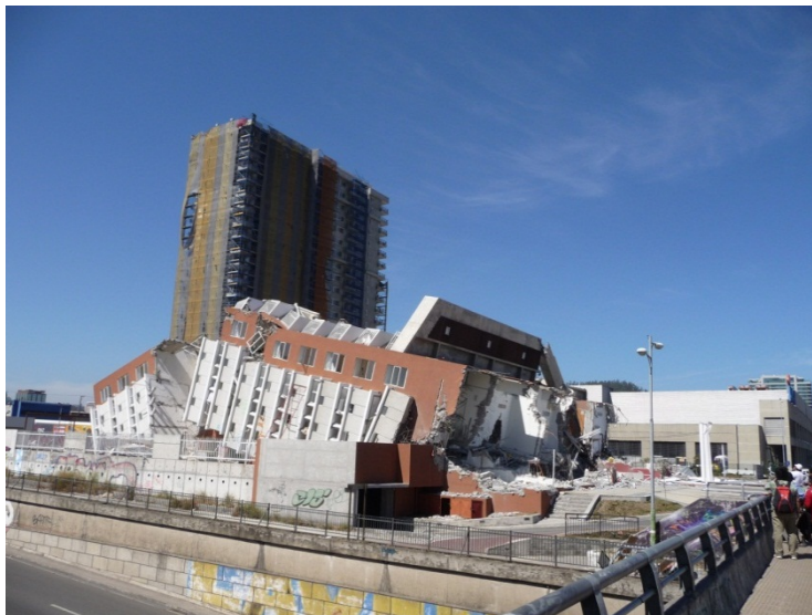
Fig. 1 – Photo of a 15 storey reinforced concrete building in Concepcion city that collapsed during 2010 Chile earthquake. (Photo courtesy of Perry Adebar)
